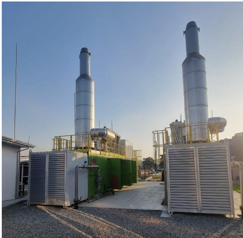
Figure 4: View of the project's electricity generation infrastructure
