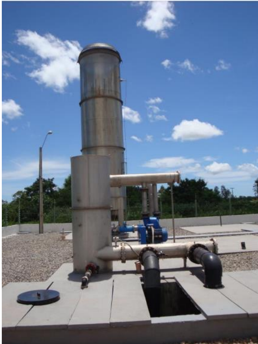
Figure 2: View of the project's LFG destruction infrastructure (flaring station)
