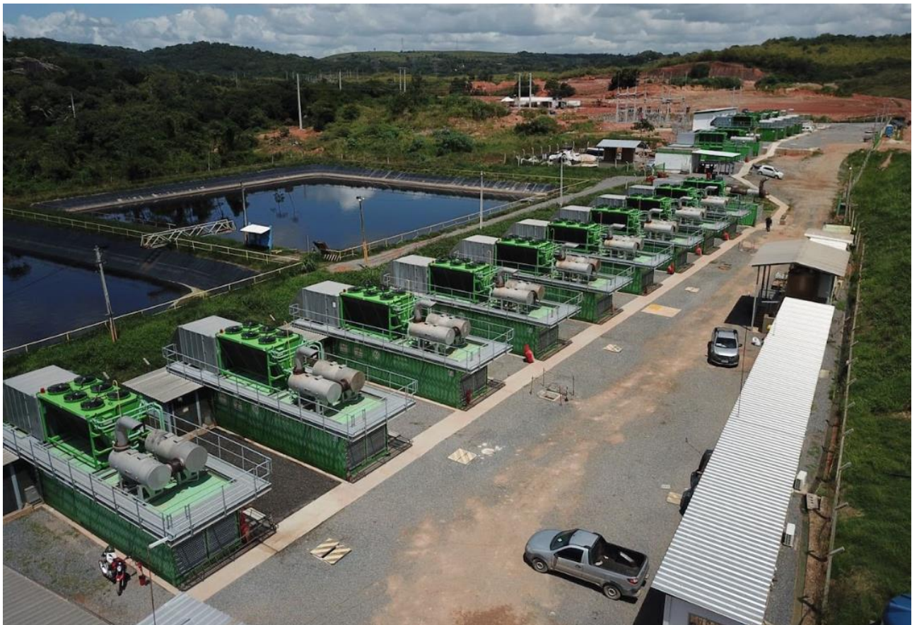
Figure 4. Picture of the engine-generator sets installed as part of the electricity generation infrastructure of the GS project activity
