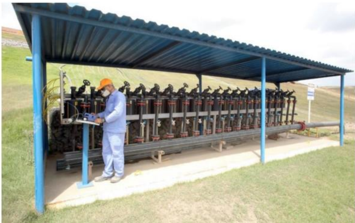
Figure 3 – Manifold in the project activity
