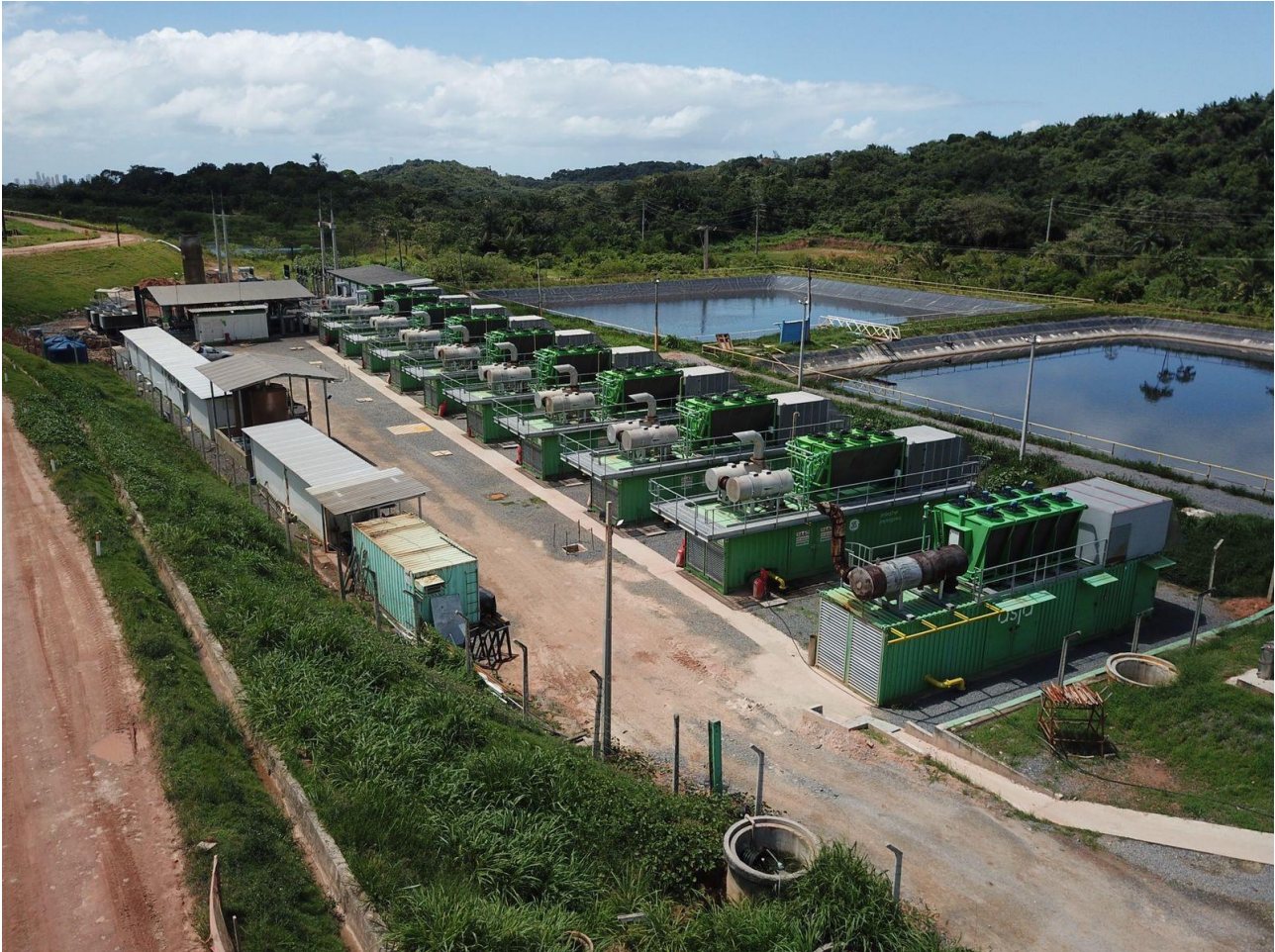
Figure 5 – LFG Engine generation units
