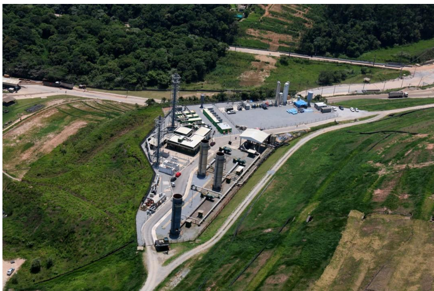
Figure 8 – Flaring station at CTL Landfill Gas Project (Source: EcoUrbis Ambiental S.A.)
