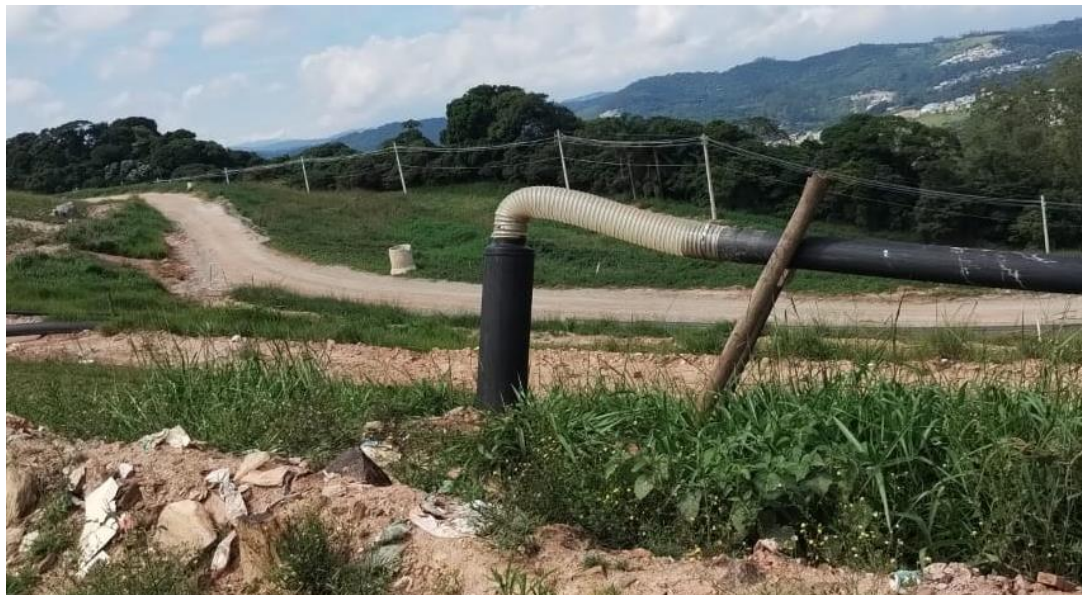
Figure 7 – Connected transmission pipelines
