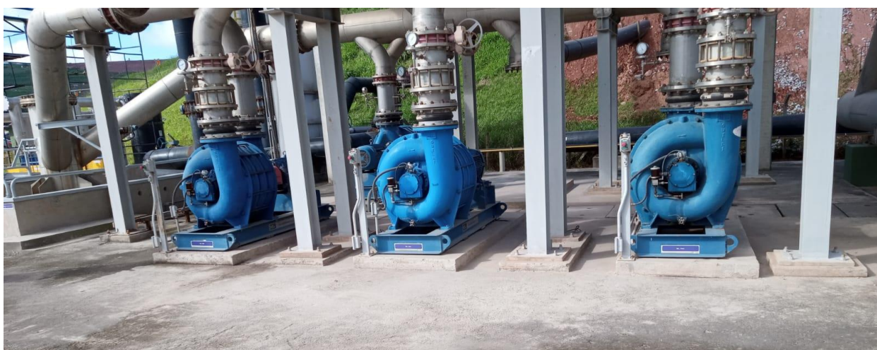
Figure 10 – Blower system at CTL Landfill Gas Project
