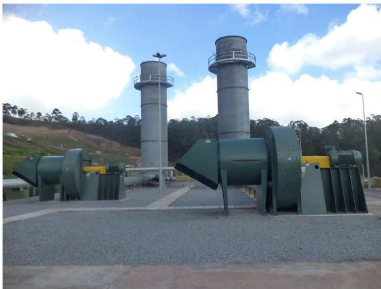
Figure 9 - Enclosed Flare system at CTL Landfill Gas Project (Source: EcoUrbis Ambiental S.A.)
