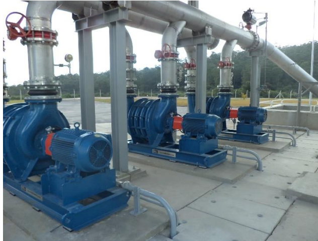
Figure 9 – Blower system at CTL Landfill Gas Project (Source: EcoUrbis Ambiental S.A.)
