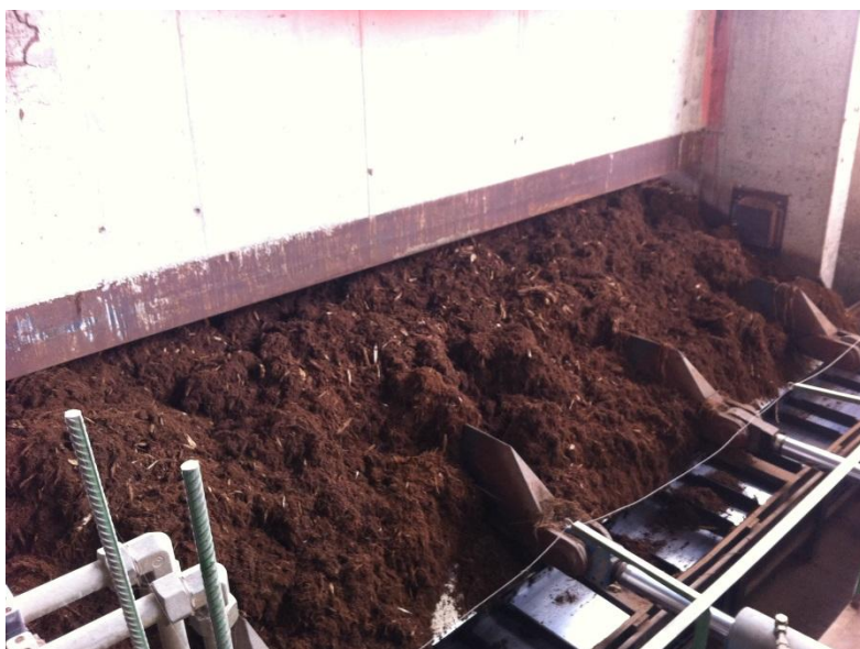
Fig. 7: Boiler fuel feeding system
