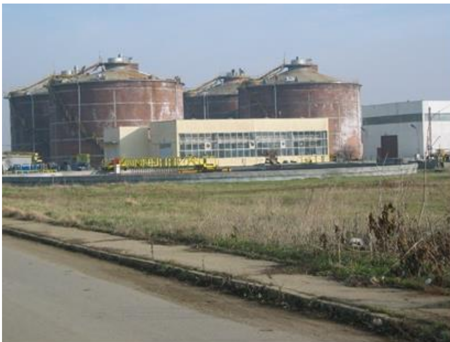
Fig.3: Digesters and raw sludge pumping house
