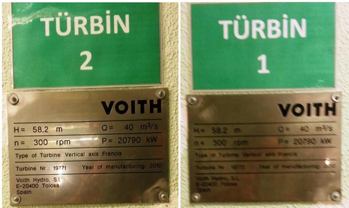
Figure 1: Nameplates of the turbines installed at the Niksar HPP, indicating the total installed capacity of the power plant (pictures are taking during the verification site visit on 27/08/2013)
