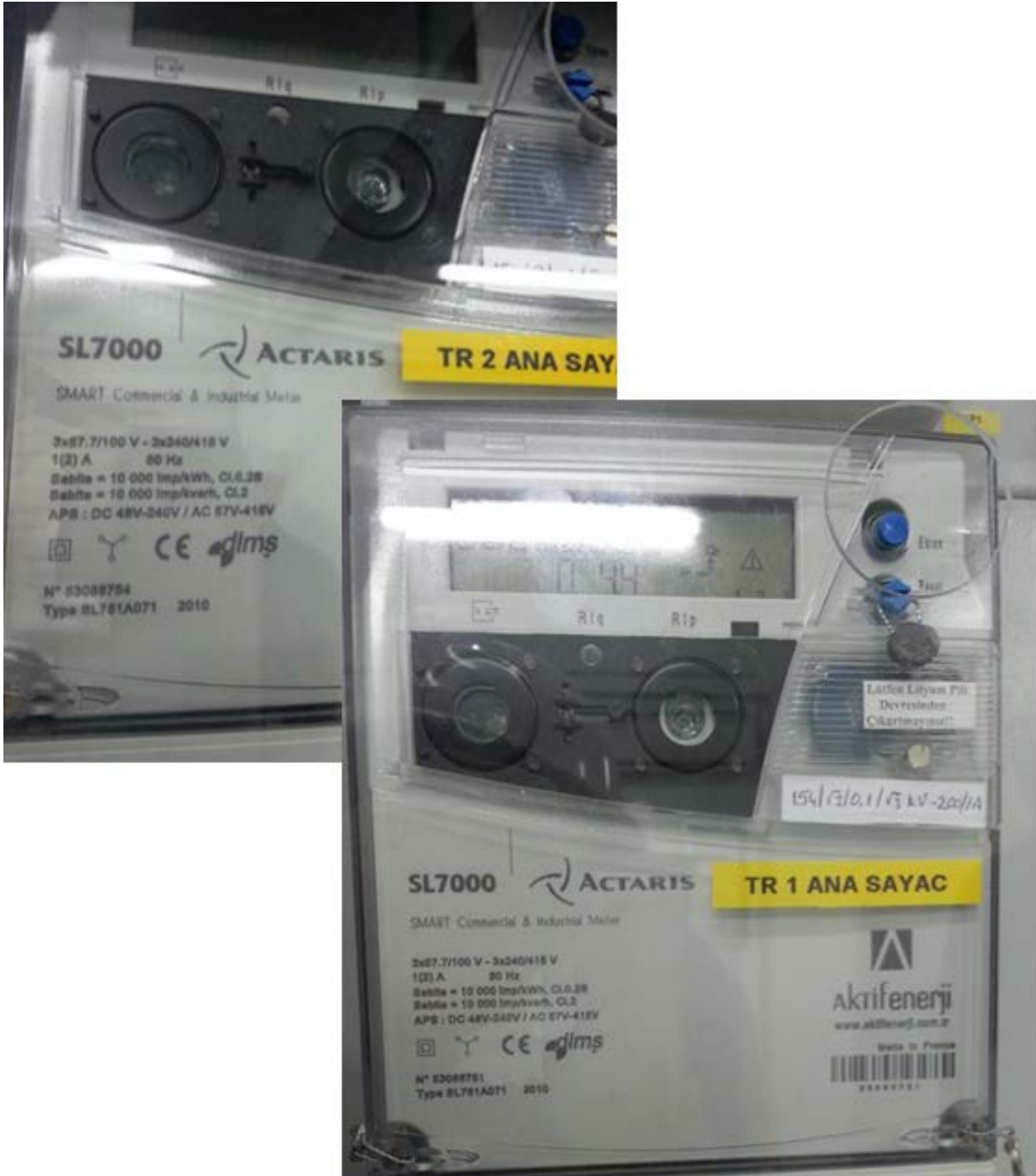
Figure 2: Main meter SN° 830887851 for transmission line 1 (TR1 right meter) and the main meter SN° 830887854 for transmission line 2 (TR2 left meter)
