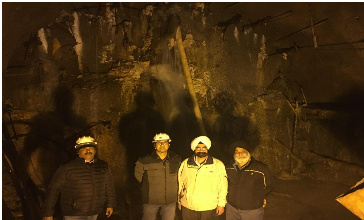
FACE-3 ABANDONED STRETCH WHERE SEEPAGE WAS FIRST OBSERVED DURING JULY,21 (seepage been channelized through pipes/ dewatering pumps)
