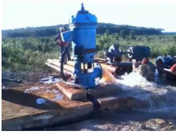
Water wells and pumps
