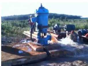
Water wells and pumps
