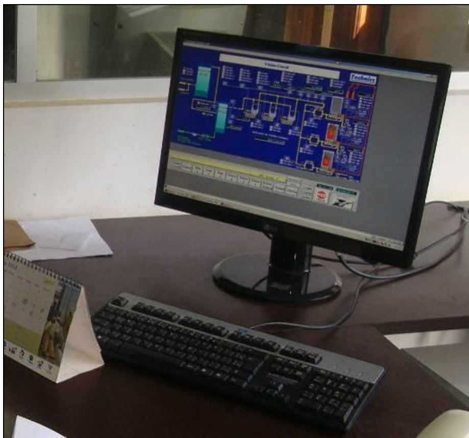
Figure 7 – PC control screen with real-time information of the operation of the LFG destruction station
