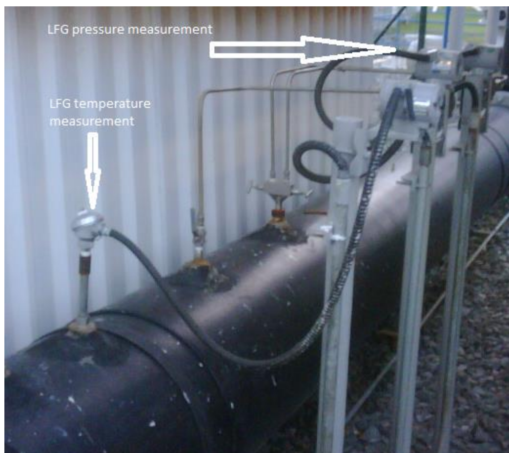
Figure 4: Location of the LFG pressure sensor and LFG temperature sensor
