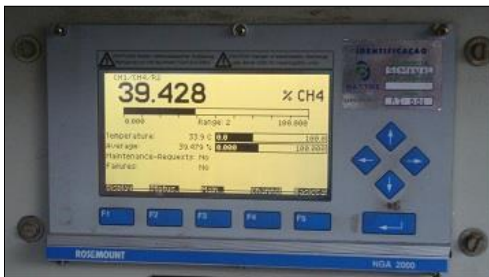
Figure 6 – Panel of the installed CH 4 /O 2 content gas analyzer unit
