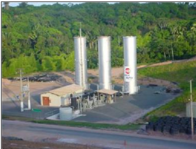
Figure 1: View of the project's LFG collection and destruction station equipped with 3 enclosed flares
