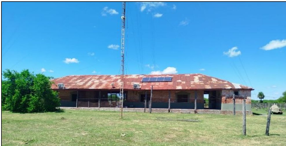
Solar Panels Installed at Visitor Center (Photo Credit: Quadriz)
