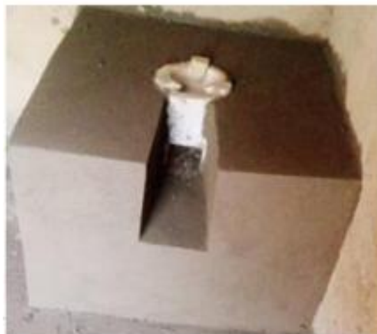
Figure 4: RDIS stove after installation
