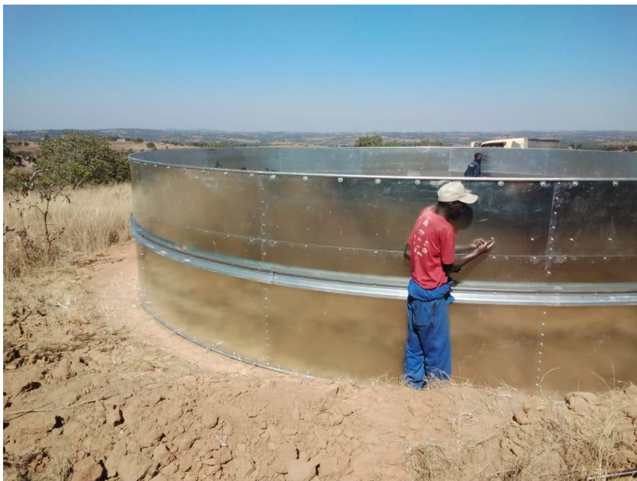
Figure 23: Kariba REDD+ Project Chinkova rainwater harvest system
