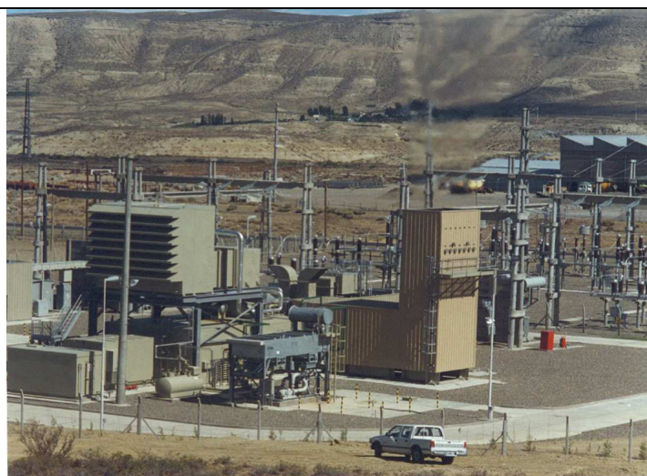
Figure 1: Central Termica Patagonia power plant
